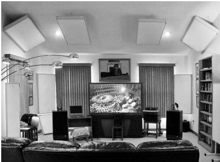
Figure 9.42d MiniTraps installed in living room.
